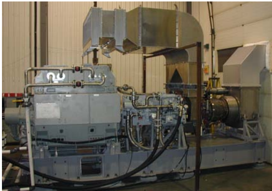
Figure 4 Gas Turbine Generator Set
